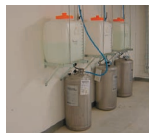
Fixed installation in car wash box.
